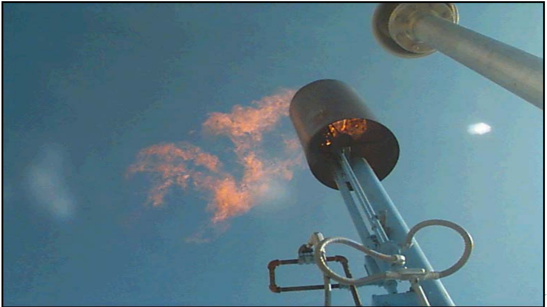
Successful production of digester gas
