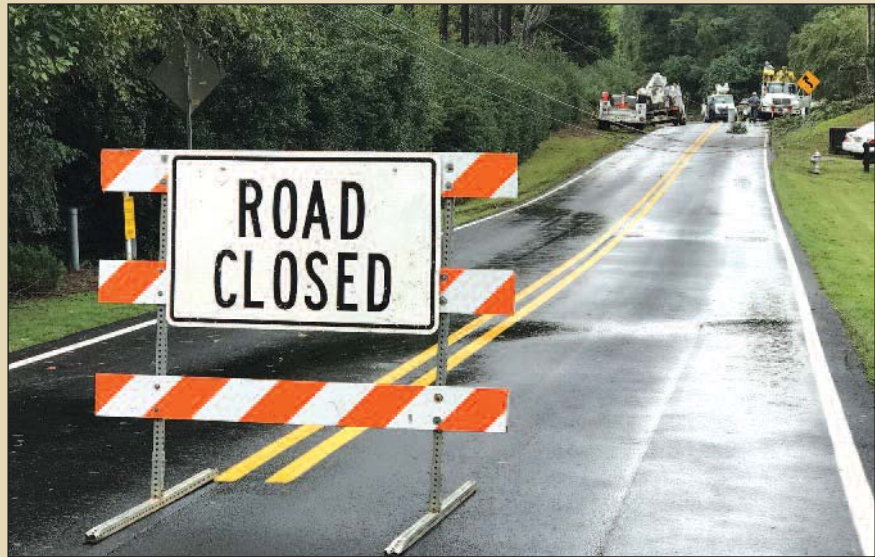
Repair crews worked around the clock to restore power in Georgia (seen here) and other parts of the country pummeled by hurricanes. Photo by Savannah Chandler, courtesy Walton EMC
