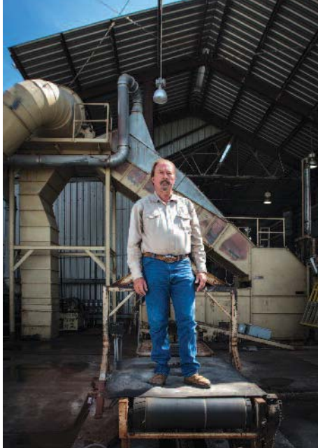
David Wyatt, manager of Bayside-Richardson Co-op Gin, stands on what is left of the seriously damaged gin in Woodsboro, Texas. Members were harvesting a bumper crop when Hurricane Harvey pounded the area, leaving multiple buildings and equipment at the gin damaged beyond repair. USDA photo by Lance Cheung
