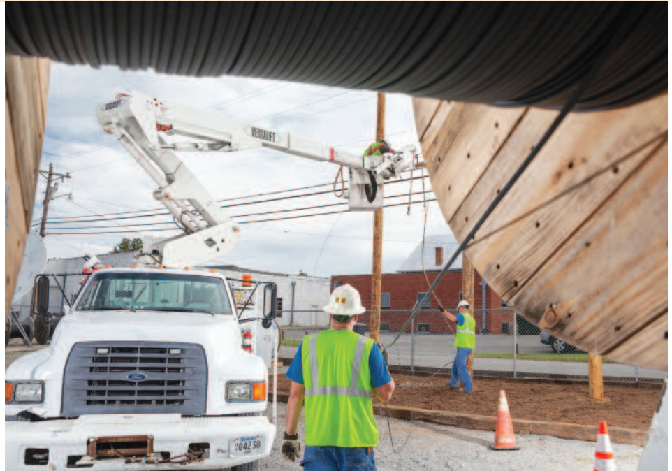
Fiber optic cable is being strung in many parts of rural Tennessee, as seen here, greatly increasing the ability of these areas to attract new, broadband-dependent jobs. Photo courtesy of Bledsoe Telephone Cooperative
