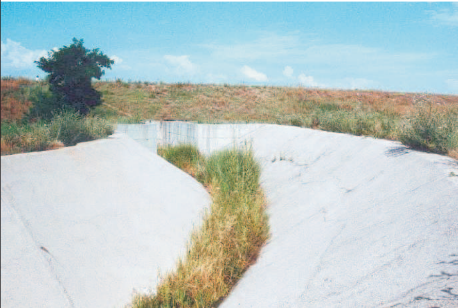
Figure 6: Overgrown Internal Canal
